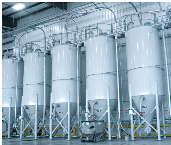
Coperion K-Tron pneumatic conveying system
